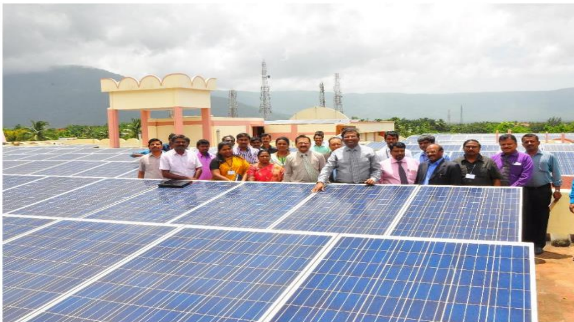
Example of Roof and water heater Solar Panels
